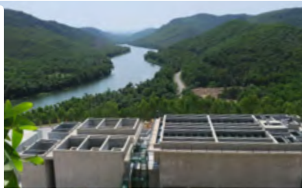
Drinking water treatment plant in Quang Binh province, Vietnam Capacity: 10,000 m 3 /d Budget: 10€ million
