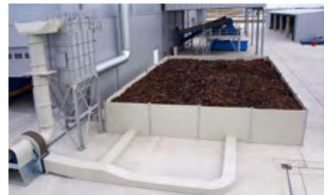
Air treatment project at a waste management centre, Subotica, Serbia Capacity: 20,000 m 3 /h
