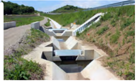
Stormwater treatment at the Lugoj-Deva highway, Romania ENVIA TRP oilseparators were installed
