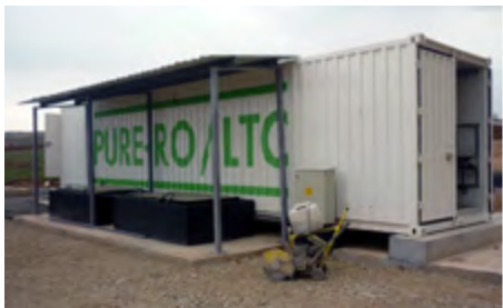
Containerized landfill leachate treatment system in Stara Zagora, Bulgaria Capacity: 150 m 3 /d
