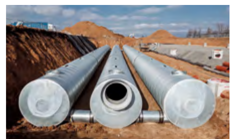
Stormwater solution for NEXEN Tire plant in Žatec (Czech Republic) 1,200 m 3 of corrugated steel pipes
